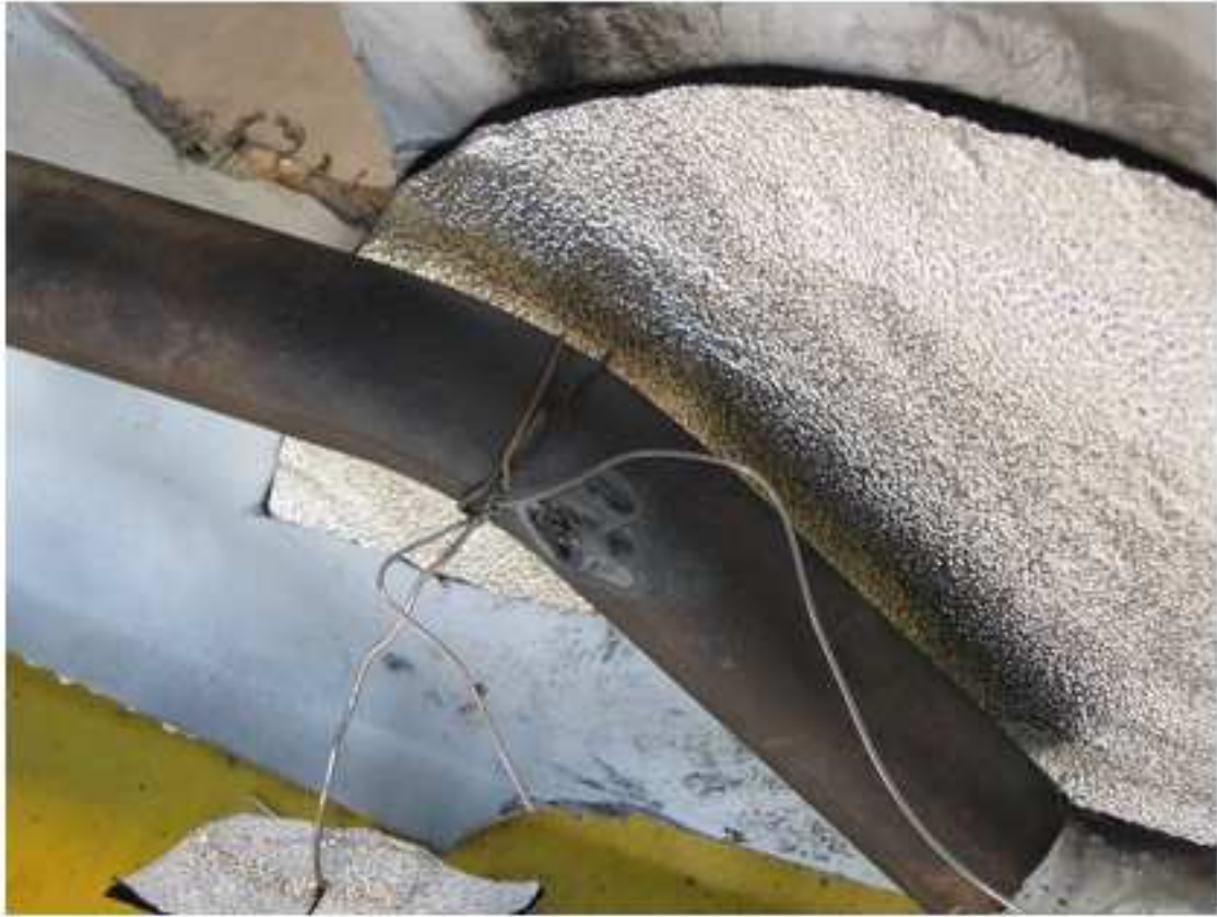
Figure 3 - Temperature measurement point on the pipe ( T_H )
